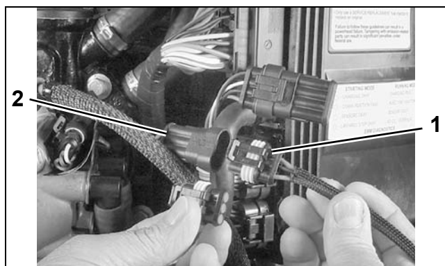
1. Water pressure transducer lead
